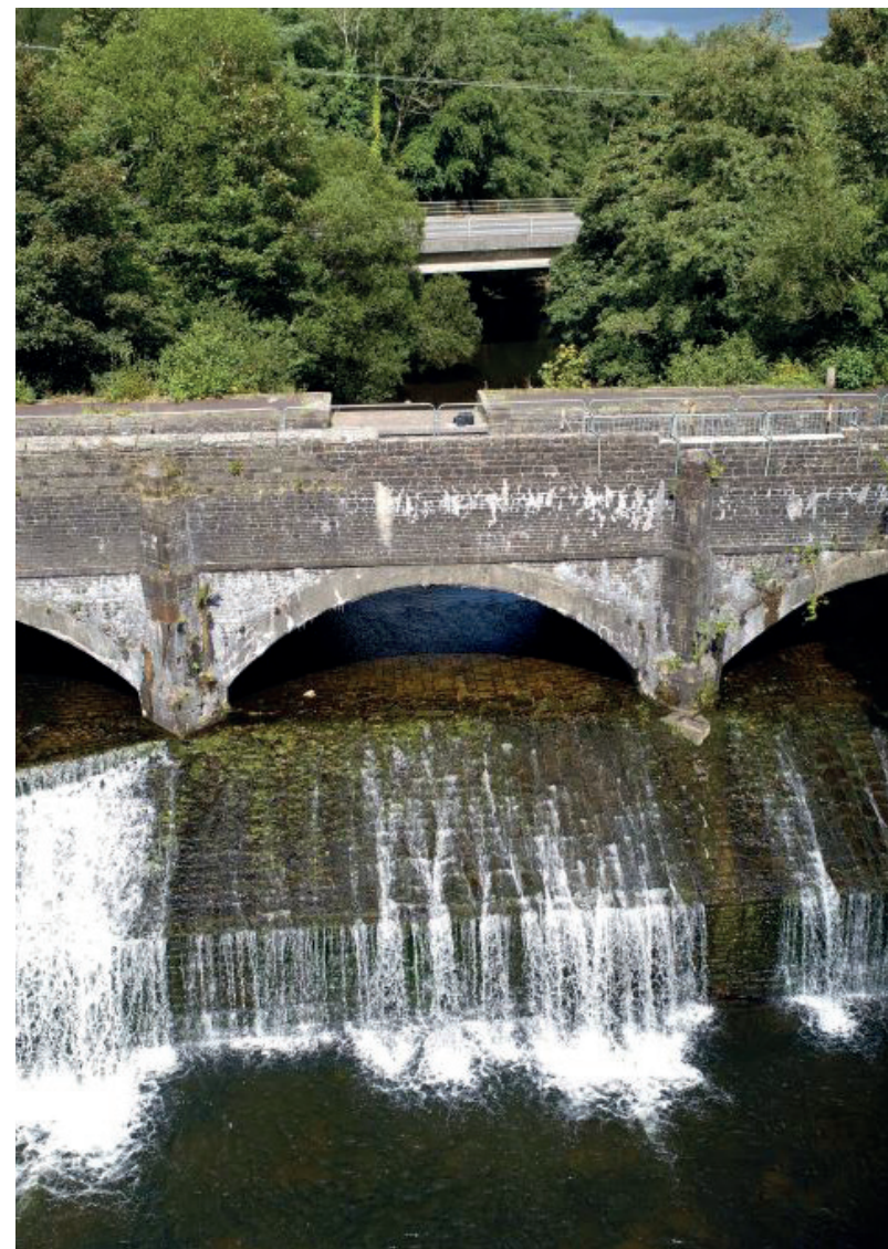
Canal Aqueduct over Afon Twrch, including weir, Ystalyfera (Grade II* Listed Building).
